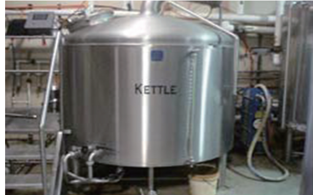
Figure 10 Kettle Heat Exchanger
