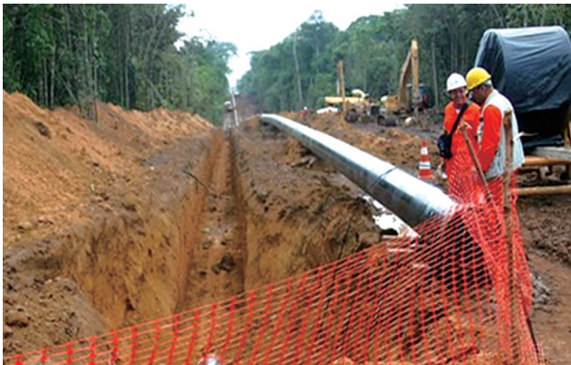
Figure 2 The Construction of the Urucu-Coari-Manaus Gas Pipeline—District of Coari, State of Amazonas 2010 (Brazil)
