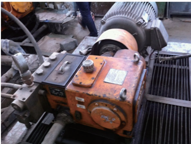
Figure 2 Pump and Three-Phase Asynchronous Motor
